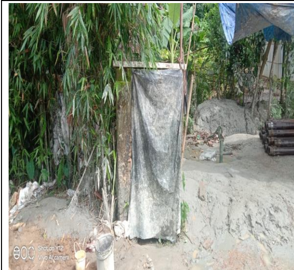
Toilet facility for workers at Mohanpur
