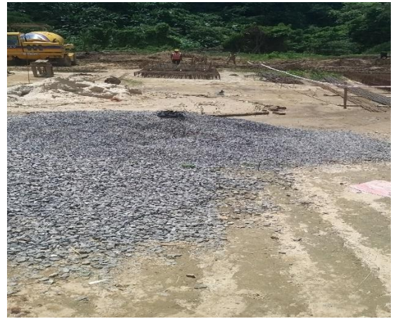
Proper material storage is required. Stone aggregates need to be removed from camp access
