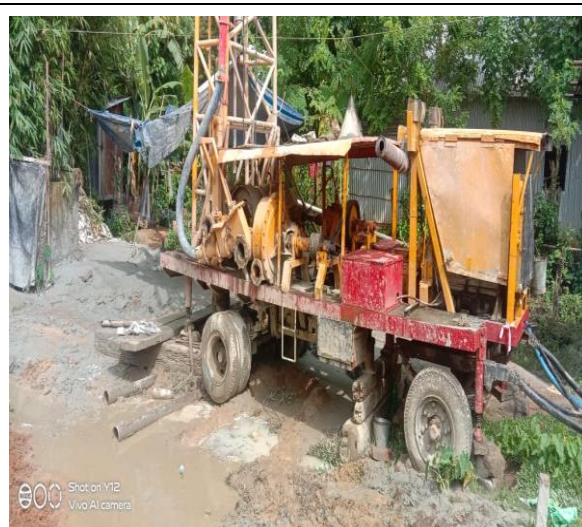
High Compressor boring machine has been installed at Mohanpur
