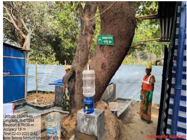
Belonia OHSR at Satmura School, provision of drinking water at site – noted
