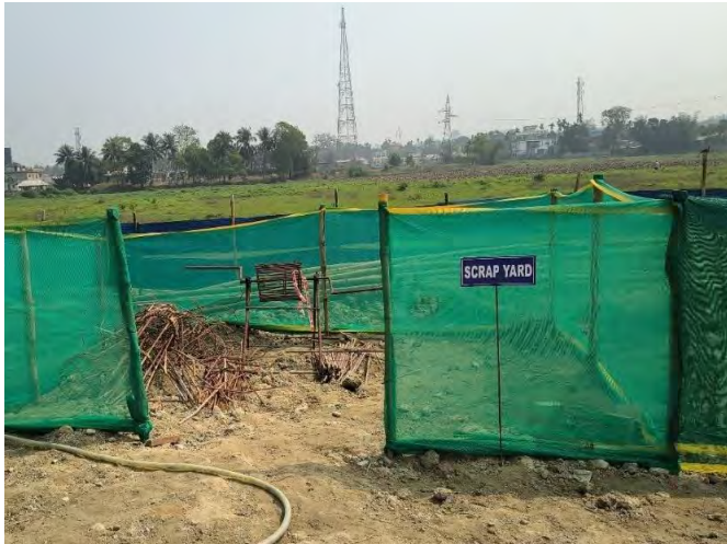
Well demarcated scrap yard at Rajarshi Town Hall OHSR, Udaipur
