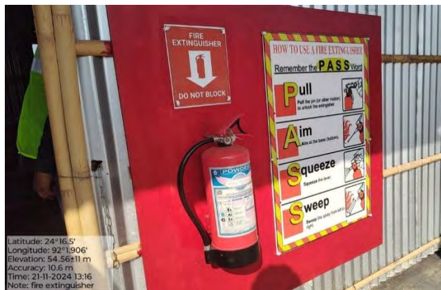
Fig. 3: Fire Extinguisher with instructions
