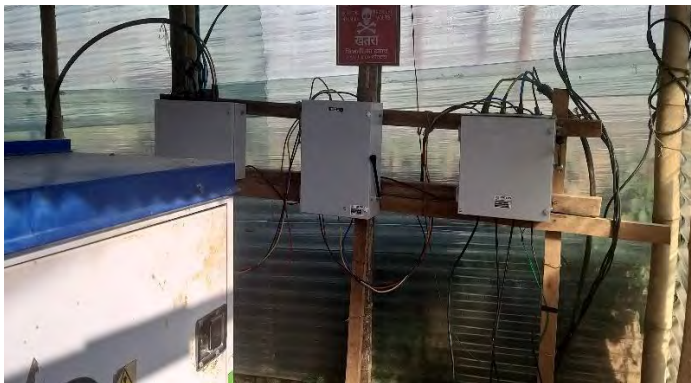
Fig. 11: Green DG placed at site. Contact no. of Electrician needs to be placed
