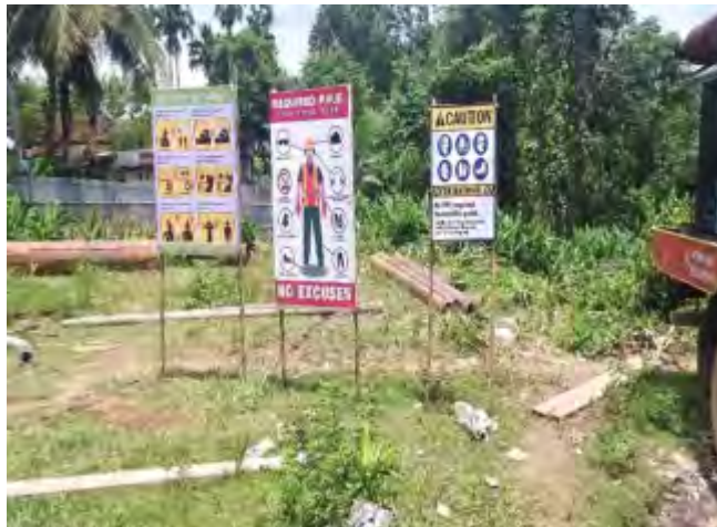
Safety signage noted at Mohanpur DTW site
