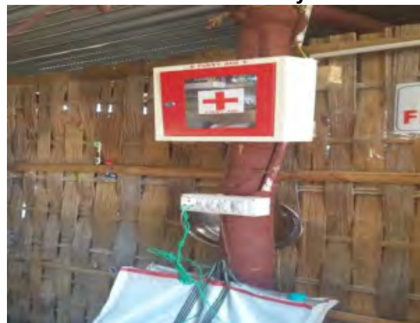
First aid box placed at labour camp
