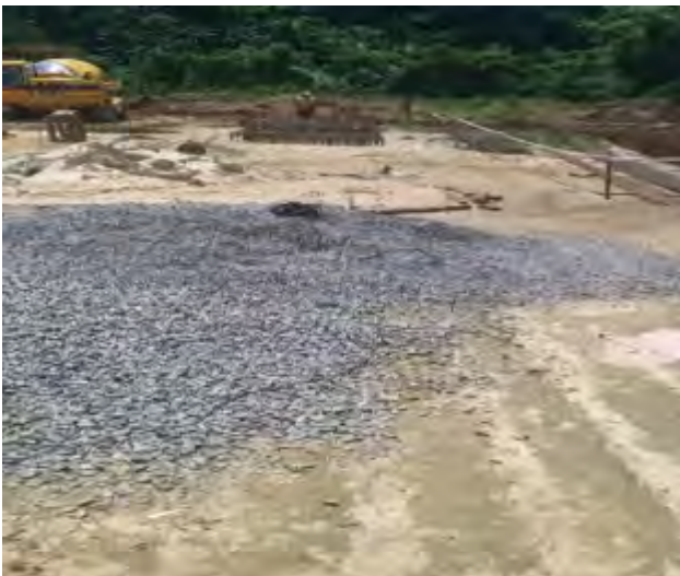
Proper material storage is required. Stone aggregates need to be removed from camp access
