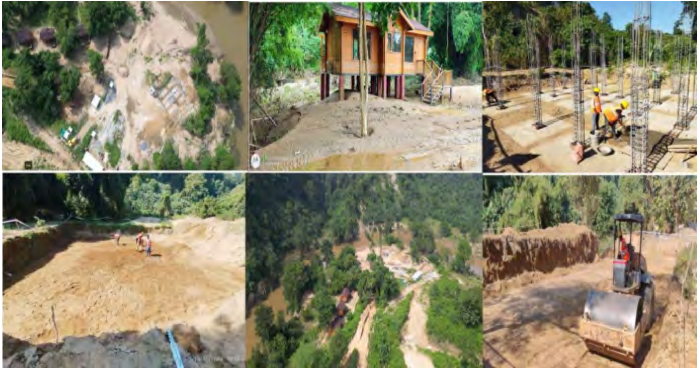
Plate 3: Pictures of Chabimura project site after the flood 2. Detail of loss due to flood (manpower/ machinery/ materials)
